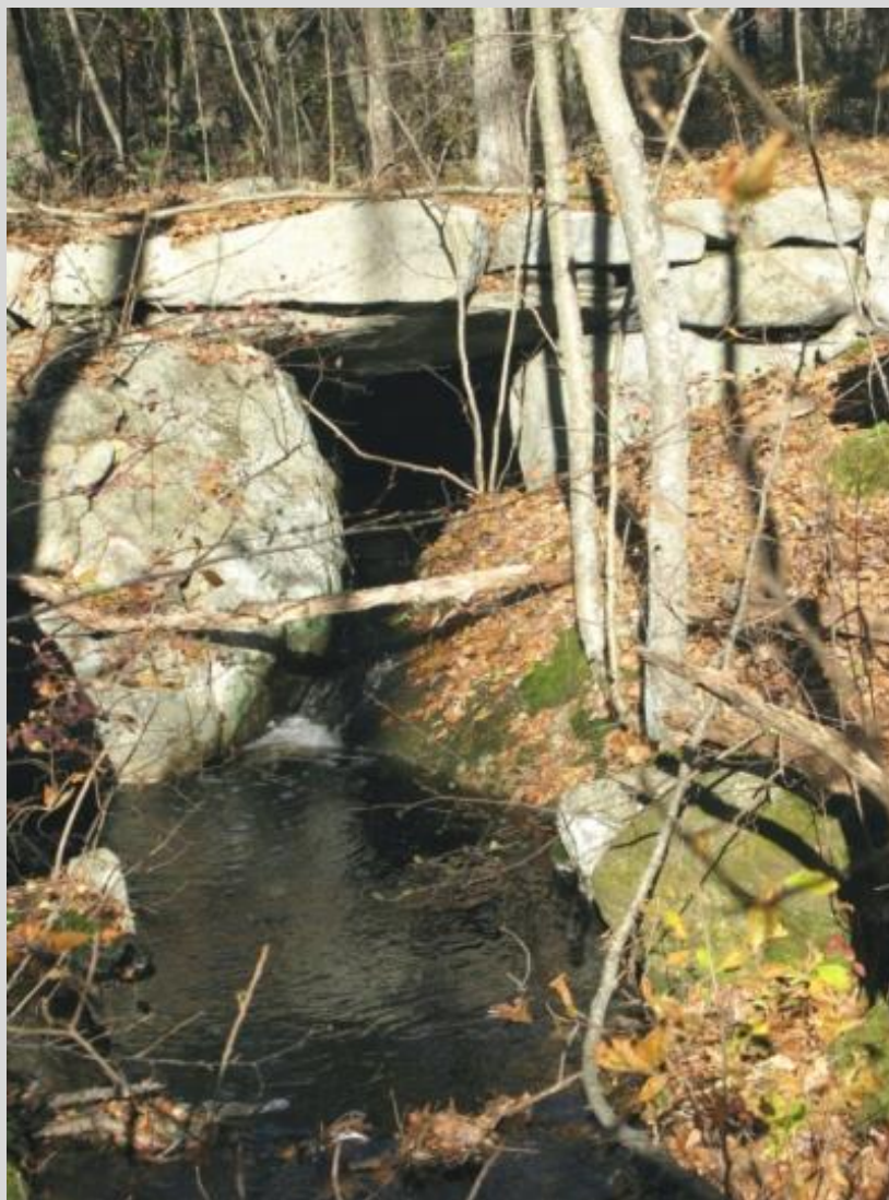
The bridge with its opening on the south side towards the mill site.
