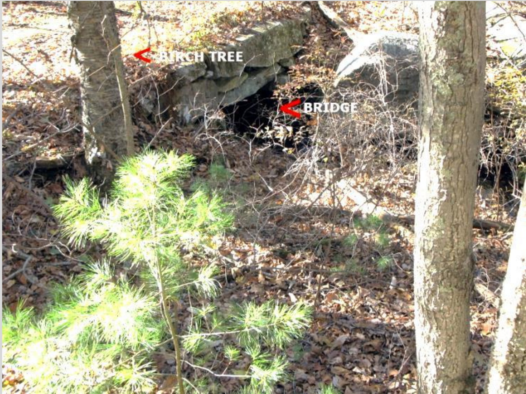
The bridge with its opening on the north side towards the swampy area which had been the pond. The old birch, which once had a tag indicating the site, is not easily recognized today.
