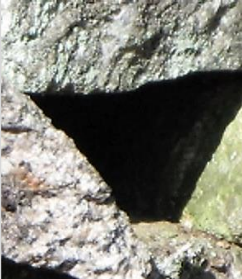
In this photo there is a triangular cut in the stone wall of the saw mill which may have held the axle to the water wheel.
